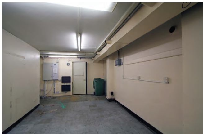
The BT equipment room
